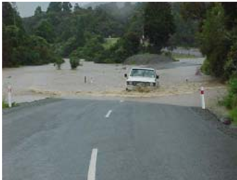
Flooding in Omoto Valley Road, Kaiata (near Greymouth) after heavy rain in 2002 made travel for residents quite hazardous. All West Coast District Councils struggle at times to keep some roads open after periods of heavy rain. Photograph from WC CDEM Collection
