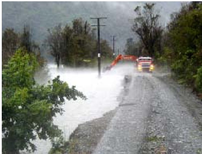
Reduction of the natural hazard risk sometimes continues as the event is occurring like this work trying to maintain the integrity of the Waiho River stop bank at Franz Josef during a flood. Photograph from WC CDEM collection.
