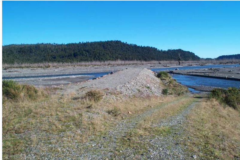
River protection works, like this rock groyne on the Waitangi-taona River, South Westland, are carried along selected rivers to prevent farm land being scoured out by floods. Photograph Wayne Moen, Engineer, WC Regional Council.
