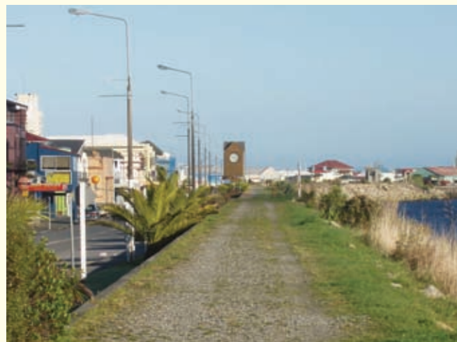
After 15 years Greymouth's floodwall is in need of maintenance. The first major flood it withstood was in 1997 but high river levels in June 2006 showed that it needs raising in places and repair in others. (Photo: M Trayes WCRC)
