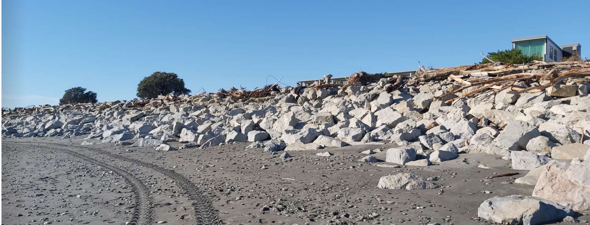
Figure 3 Existing 2013 revetment showing rock breakage, rock displacement, profile and debris line near crest
