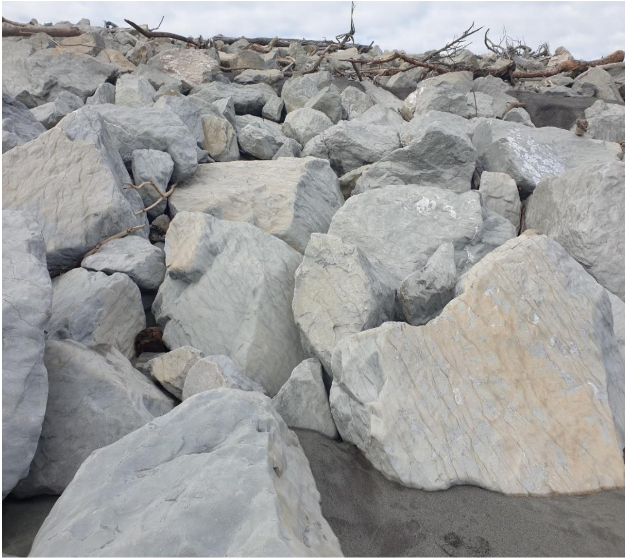
Plate 5: Existing seawall (May 2021), Hokitika Beach. Not suitable for blue penguin due to steep angle and hole size between boulders.
