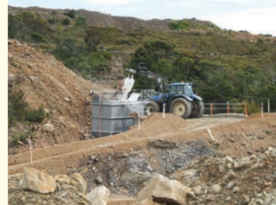
Solid Energy staff top up the lime dosing plant by the haul road above the Mangatini River. The finely ground lime is added to the river water to neutralise acid water which drains from the opencast mine workings
