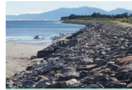
In 1998 ratepayers at Okuru became concerned by increasing erosion near their properties on the landward side of the Okuru River estuary. After advice from the Regional Council a Rating District was formed and this rock protection work was erected in 2000 to help prevent further erosion. [Photo: M Traves]
