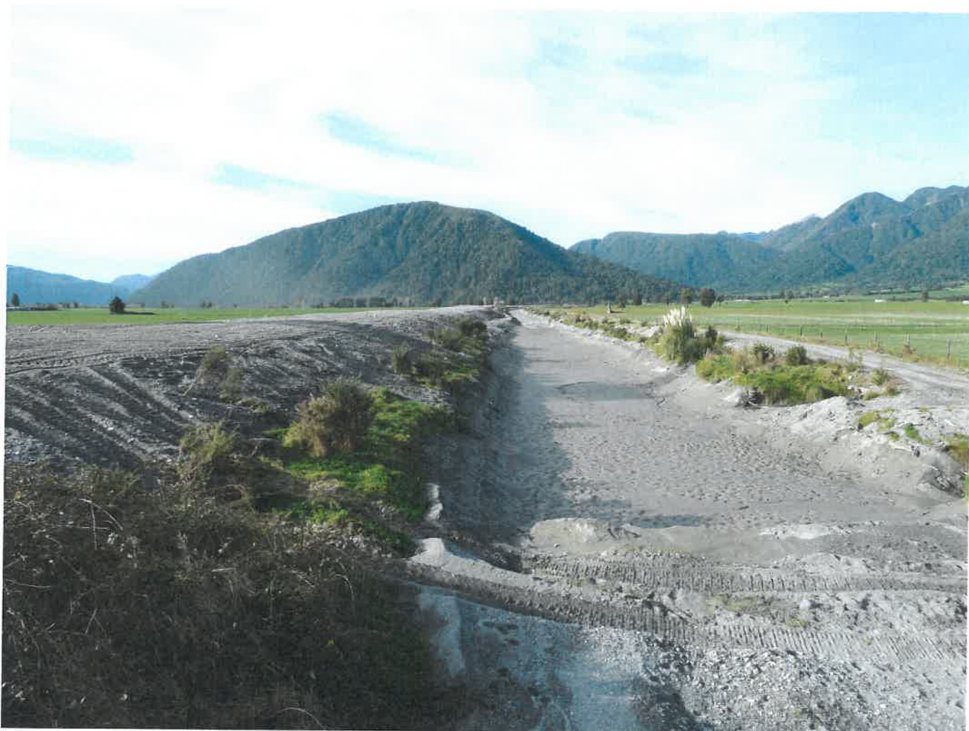
Vine Creek Rating District – Looking Upstream From Main Road Bridge Final Channel Cleanout & Leveled Spoil – May 2013
