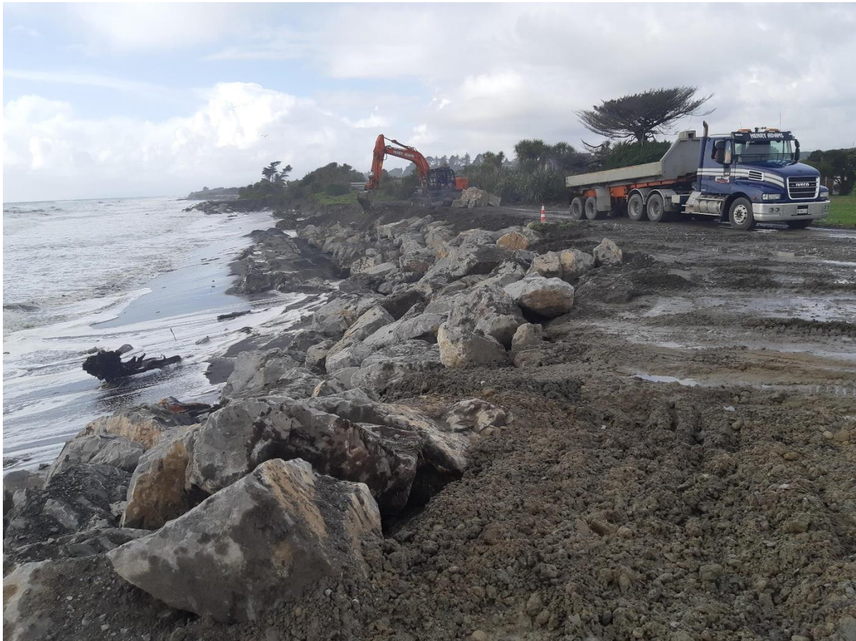
Henry Adams Contracting placing rock on 24/08/2020 (first day of works). Hampden Street groyne is visible in the distance.
