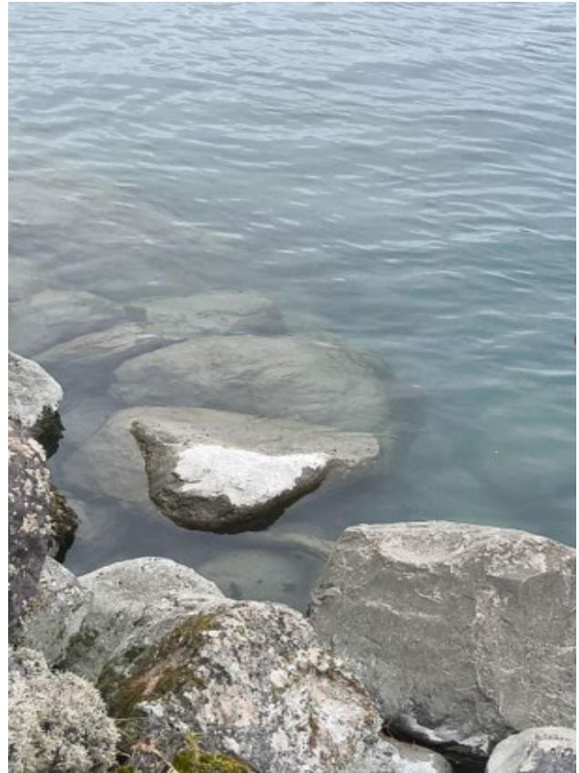
Figure 6: Wanganui River – slumped rock at base of rip rap
