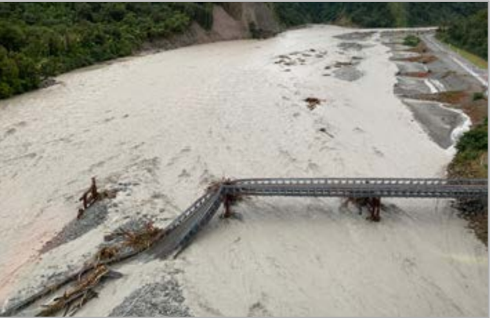
Bridge loss, 2019 severe weather (Photo credit: WCEM)
