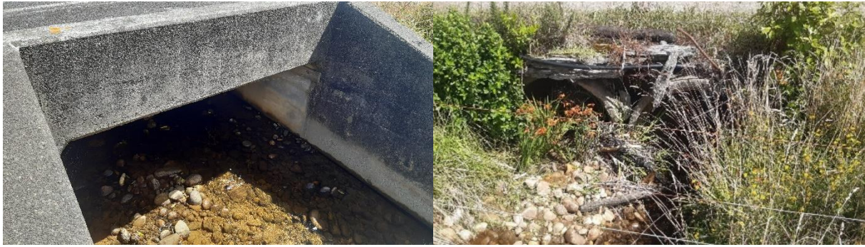
Figure 2-7: Culverts on Chatterbox Stream. Left photo: State highway bridge/culvert. Right photo: twin barrel farm culvert immediately downstream of highway. During the February 2022 flood, the farm culvert blocked and caused water to spill into the Township Catchment.
