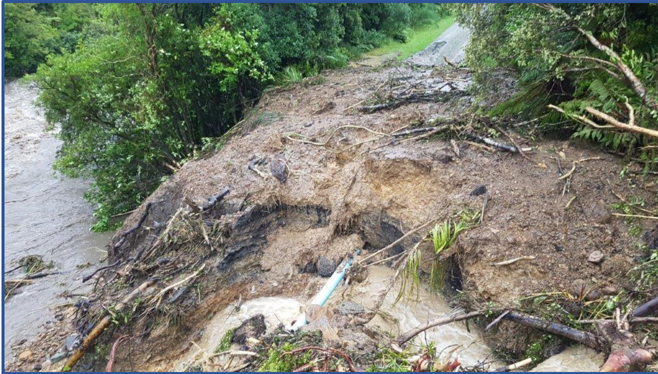
Conn's Creek slip, 10 February 2022
