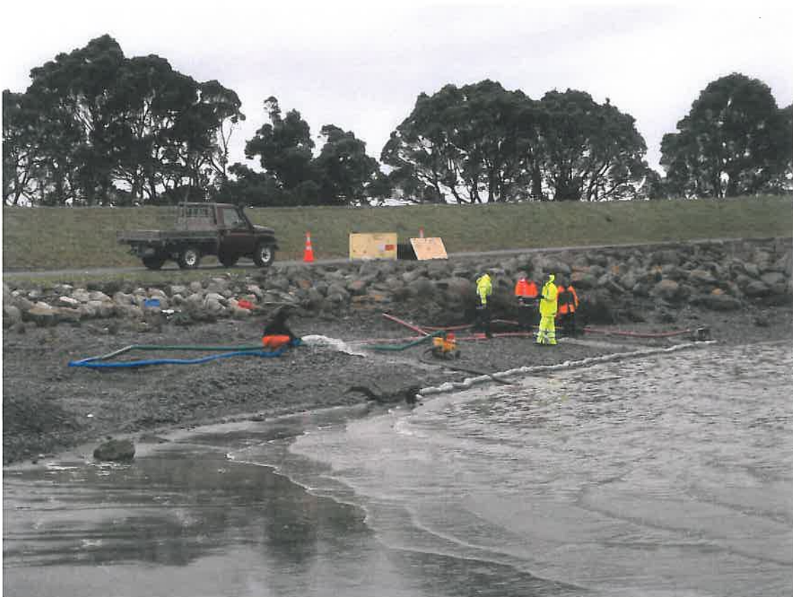
Staff operating the pumps on foreshore
