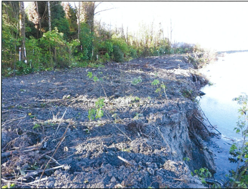
Site has been cleared of trees and scrub with the trees and scrub buried to form the base for an access road along the river bank.
