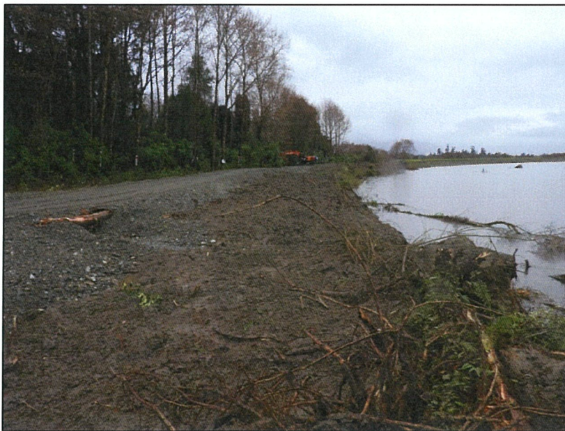
Access Road has been completed using imported gravels as well as installation of two temporary culverts.
