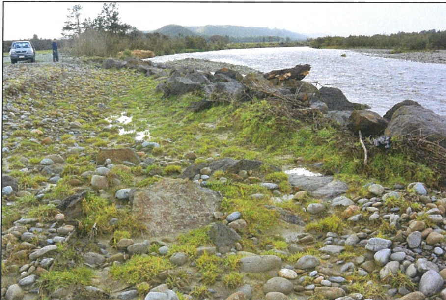
Scour behind rock groyne, Nelson Creek.
