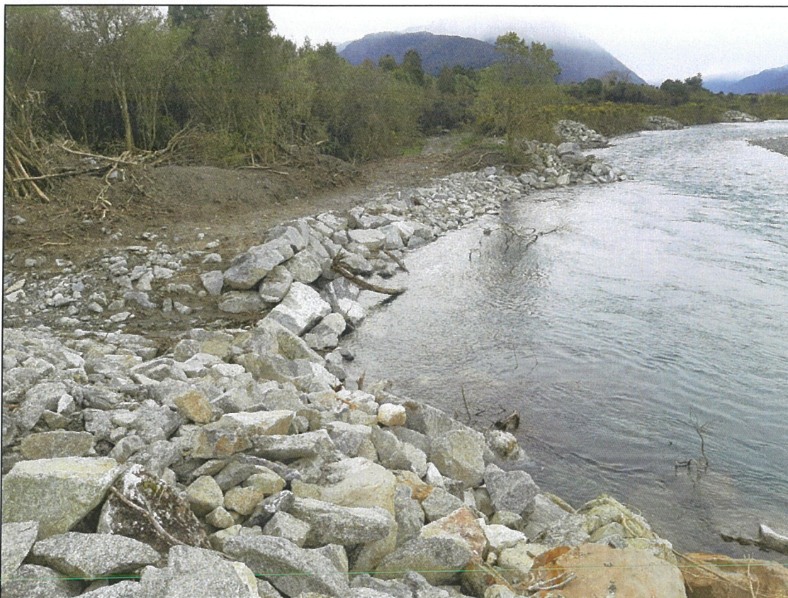
Completed Rock Riprap – Where large hole had formed
