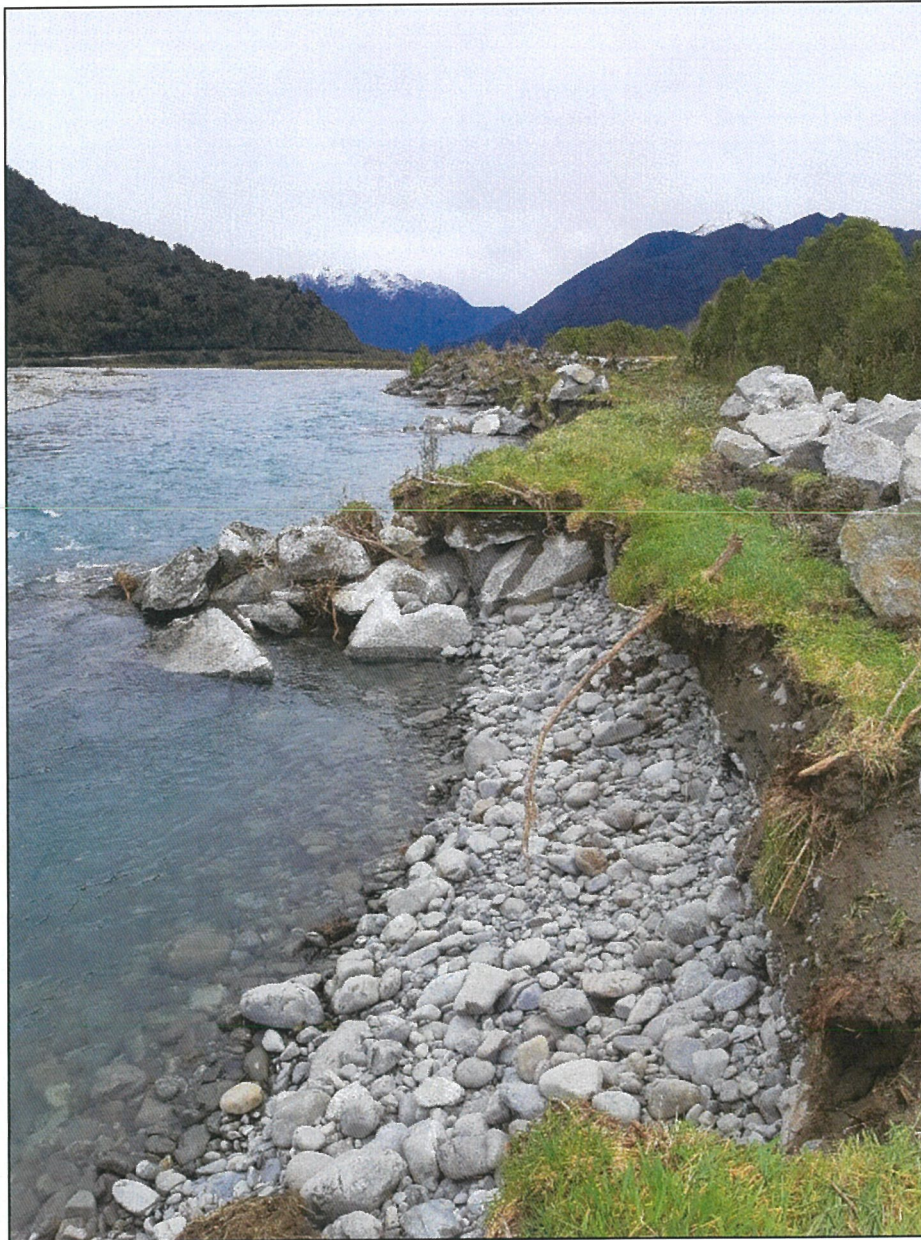
Erosion between groyne
