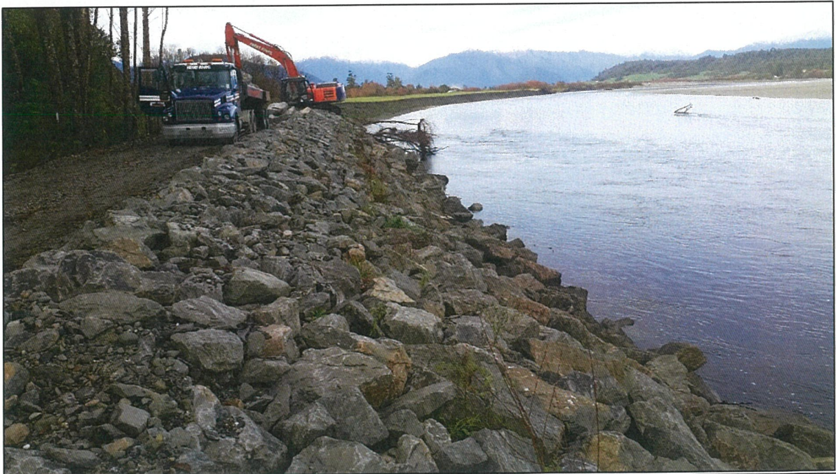
Placement of rock at slumped areas of the rock riprap at Kaniere
