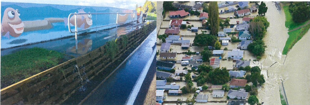
Figure 1 – The College Road Floodwall at Edgecumbe at 0841hrs on 6 April 2017. Structural failure of the wall occurred at approximately 0830hrs
