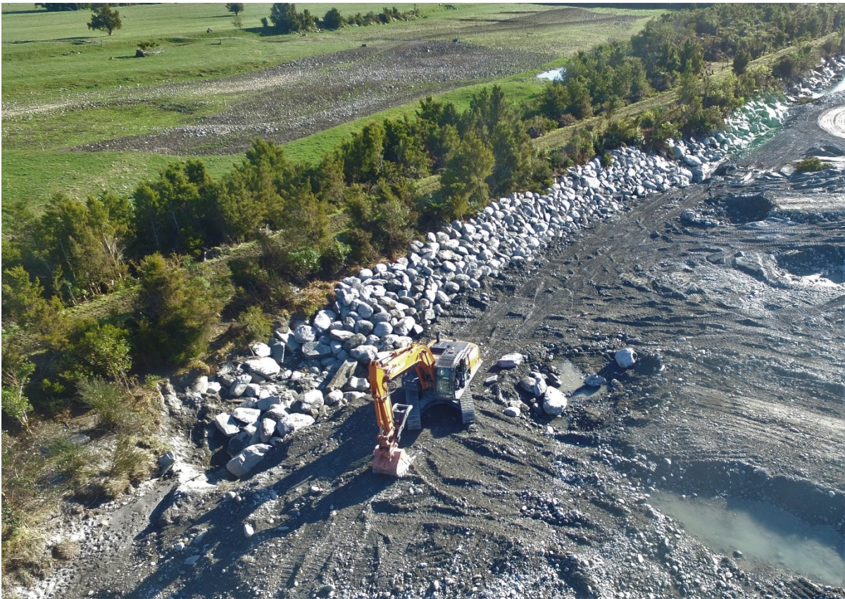
McKenzie Contracting operator awaiting the delivery of rock to be placed along the tail of the hook groyne
