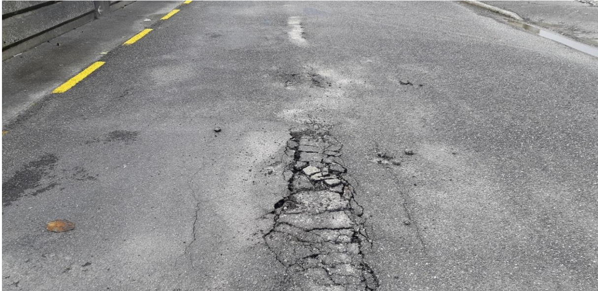
19 th July 2021. Damaged road seal due to seepage pressure on Richmond Quay.
