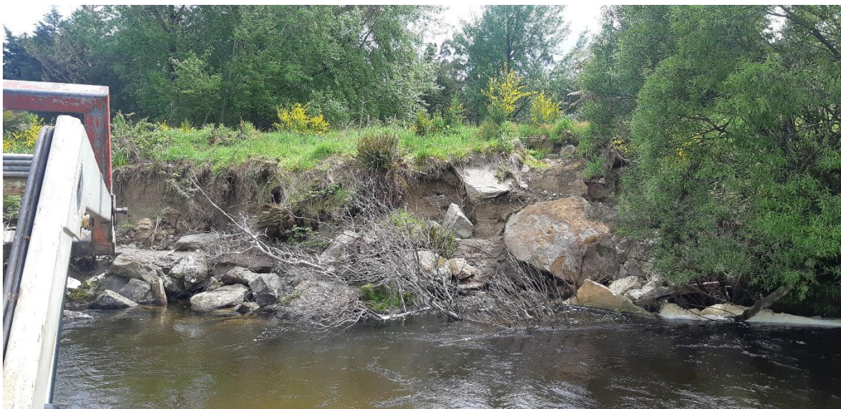
Photo 1: Erosion of stopbank batter 130m upstream of road bridge.
