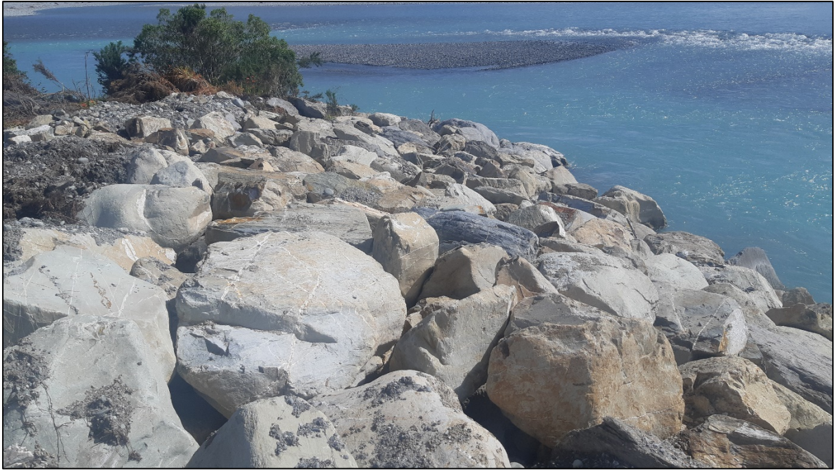
Completed maintenance work to rock along the tail of a hook groyne opposite Blackburn's Boundary
