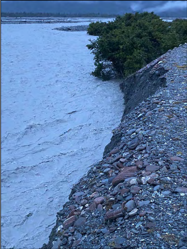
Damage to Stop bank
