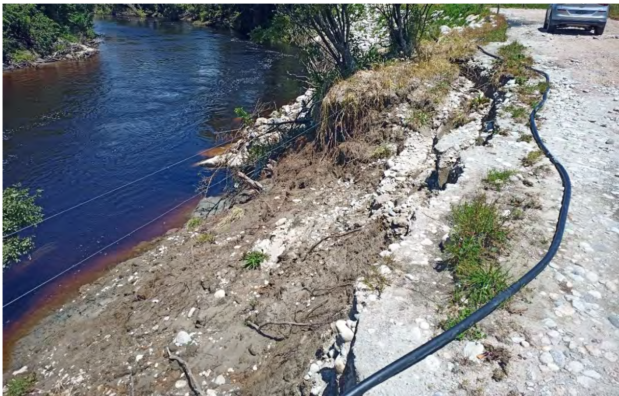
Photo 2: Looking down stream along slumped riverbank
