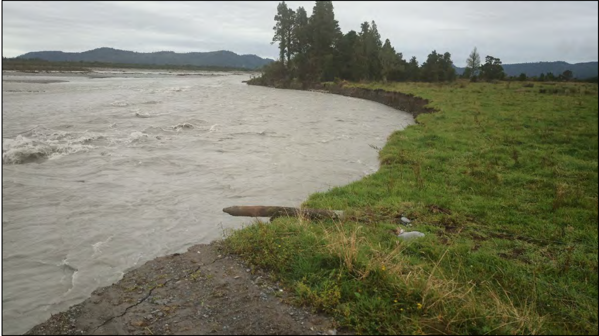
Downstream view of erosion damage
