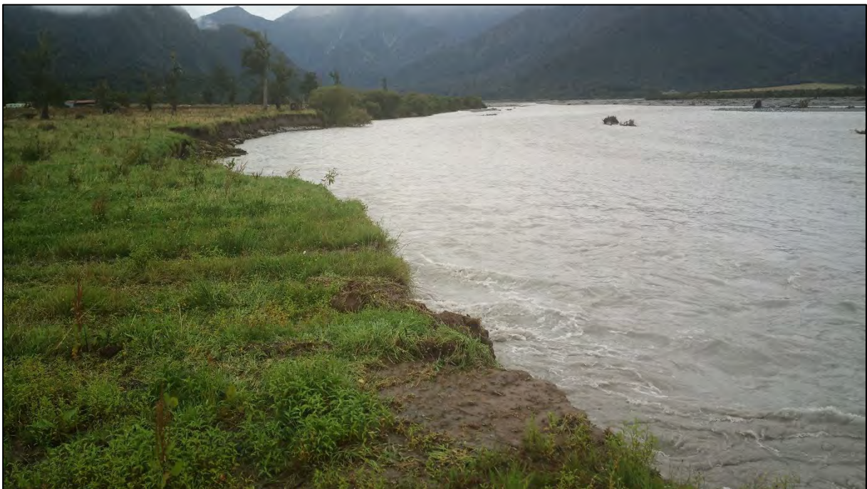
Upstream view of erosion damage
