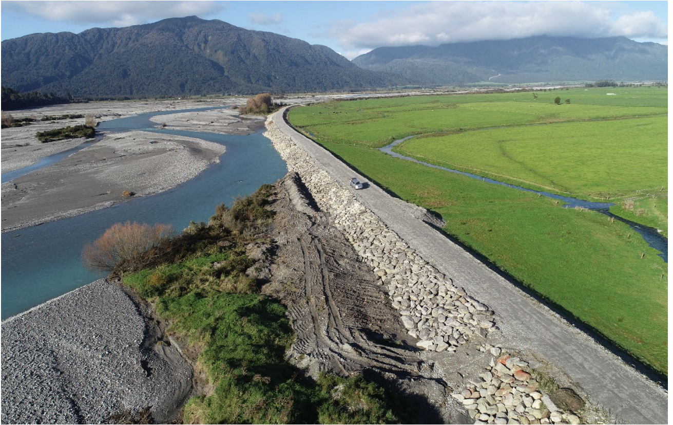
Image: Repaired and rock riprapped stop bank on the true left of the Wanganui River
