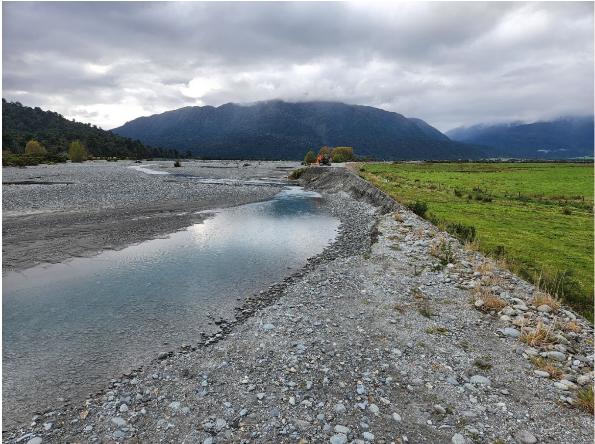
Image: Damage to stop bank before repair works started
