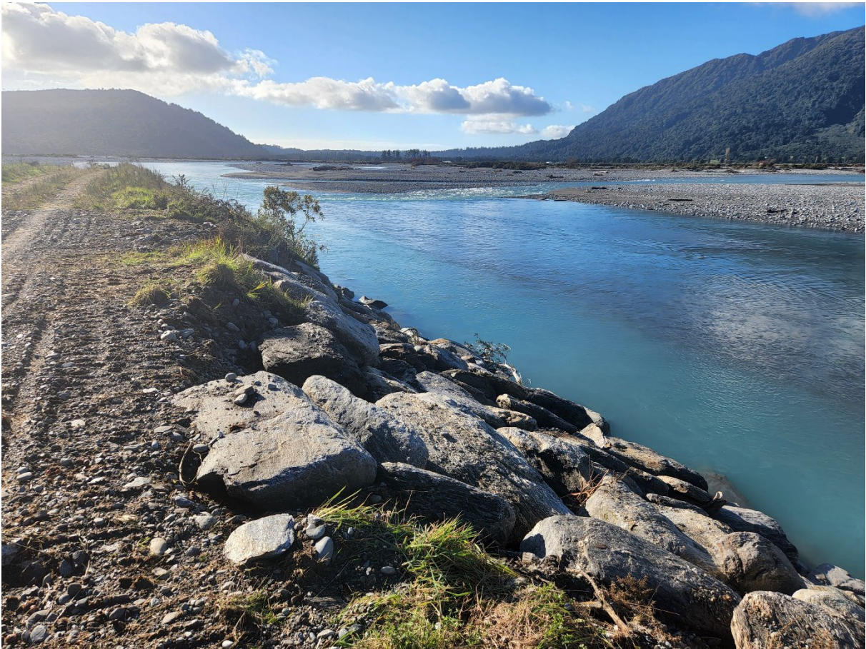
Image: repaired section of riprap on the tail of a large hook groyne
