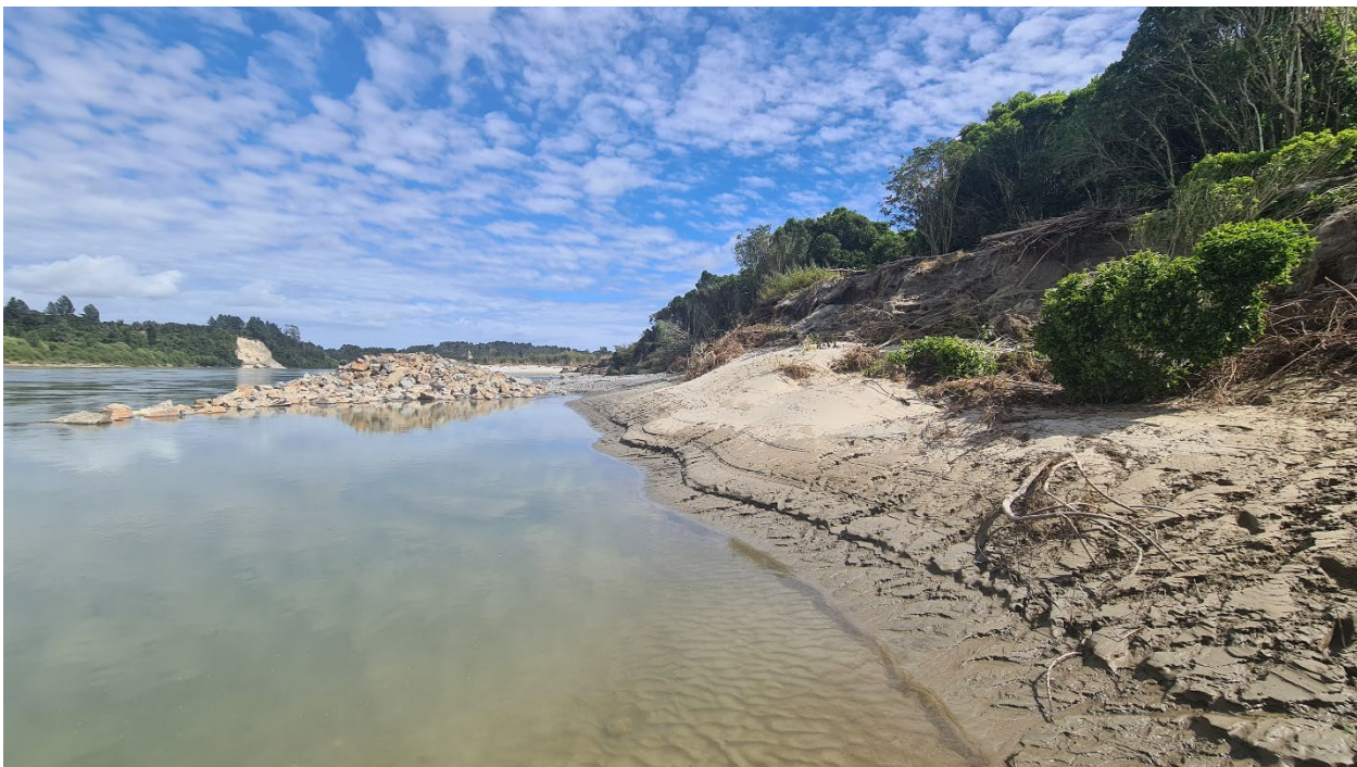
Figure 7: Looking downstream showing erosion of bank and scour behind rock training wall
