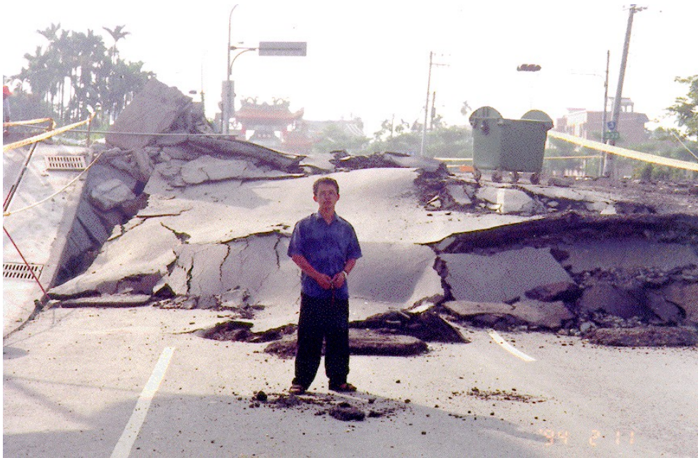
Figure 8 Photograph taken of a surface rupture related to the 1999 Chi-Chi earthquake fault, Taiwan. The view is looking toward the fault, which has ruptured through a road. The man is standing on the footwall side of the fault. The hangingwall has been overthrust and warped over and across the footwall block toward the camera.
