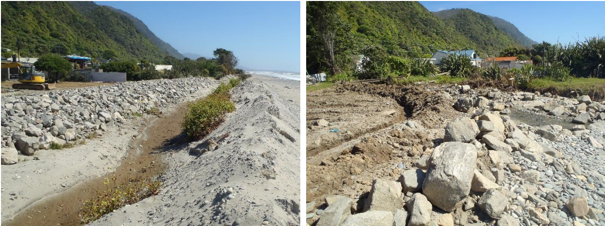
Figure 4 Recent hard defences under construction north of Bradley Stream (G4) where the drain diversion bund failed. Left, 158-160 Torea St; Right, 154 Torea St. [Source: M Allis 22-11-2016].
