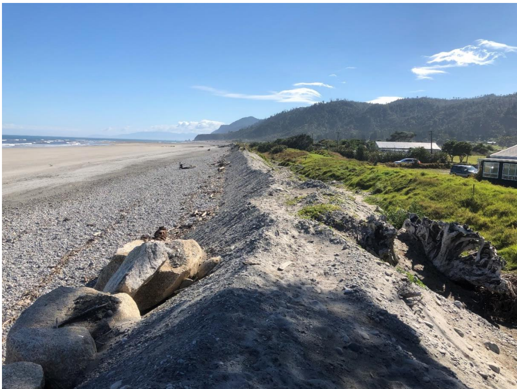
Figure 3-5: Double bund fronting Mokihinui township. Note steep (at angle-of-repose) seaward face of seaward bund, cobble ramp on upper foreshore, and wide sandy lower foreshore.
