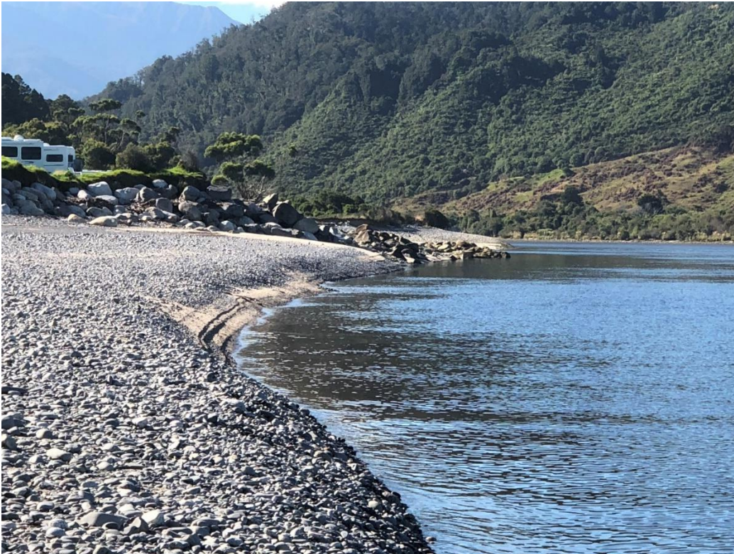
Figure 3-1: View upstream on north bank to the root of the training wall. Rock riprap in front of campervans has partially collapsed.
