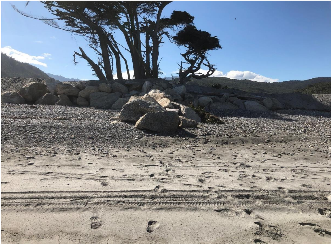
Figure 3-6: The spur groyne south of Lewis Street. Note no difference in width of cobble ramp either side.
