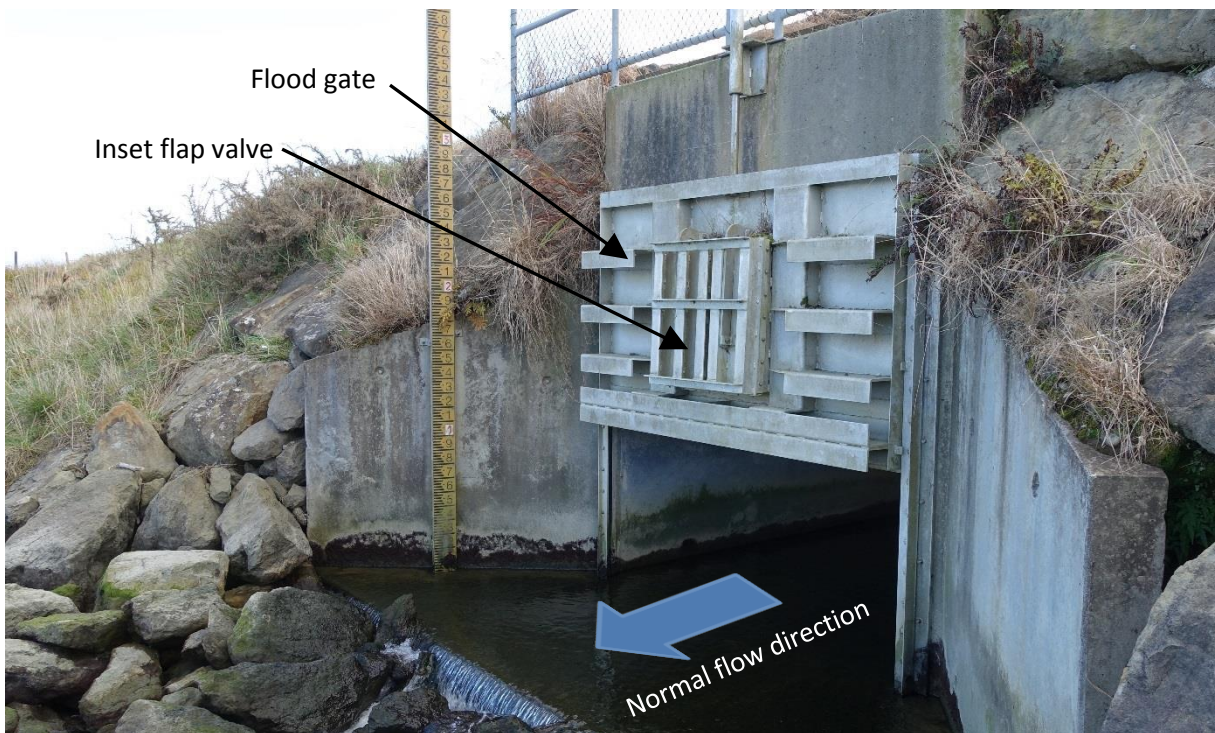
Figure 2-10: Downstream end of Cobden Lagoon outlet culvert. 2 m by 1 m rectangular culvert through Grey River stopbank with vertical sliding flood gate which is manually closed during Grey River floods. Note smaller flap gate inset into flood gate.
