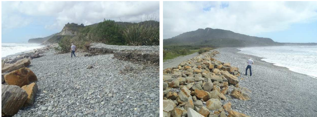
Figure 3-3: Continued erosion behind the rock revetment along the former Beach Rd between Morpeth St and Holland St (left) and recent protection works alongside Beach Rd south from Statham St (Right). Left: note former Beach Rd tar seal and basecourse layers at right of image. [Credit: M. Allis].
