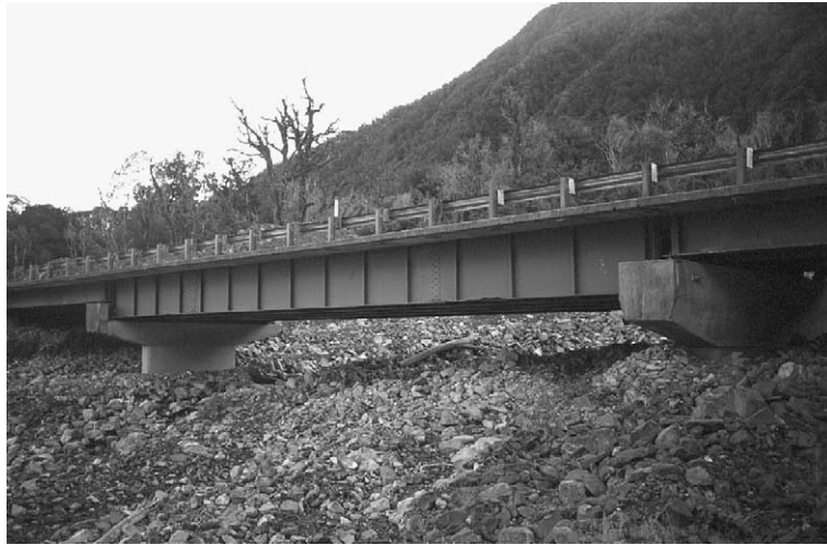
Fig. 10. Massive in-channel aggradation on Boulder Creek at State Highway 6 bridge (March 2002). Overloading of channels by coarse landslide-derived sediment continues to be a problem to infrastructure long after the causative slope failure. River flow is from right to left.
