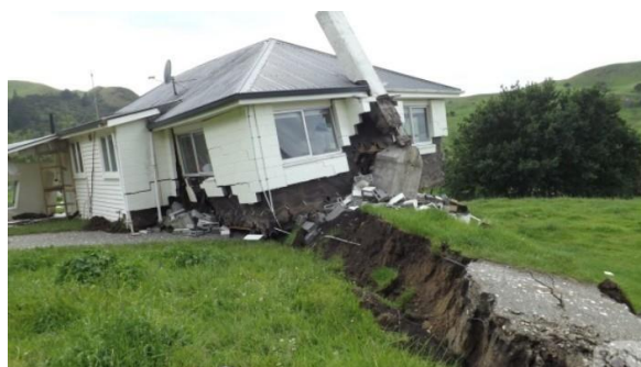
Figure 15-18: Dwelling impact directly by fault rupture, Kaikoura, November 2016 (stuff.co.nz after GNS)
