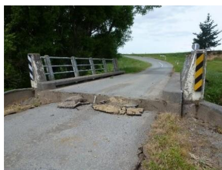
Figure 15-16: Example of a bridge approach which has settled and impeded access temporarily
