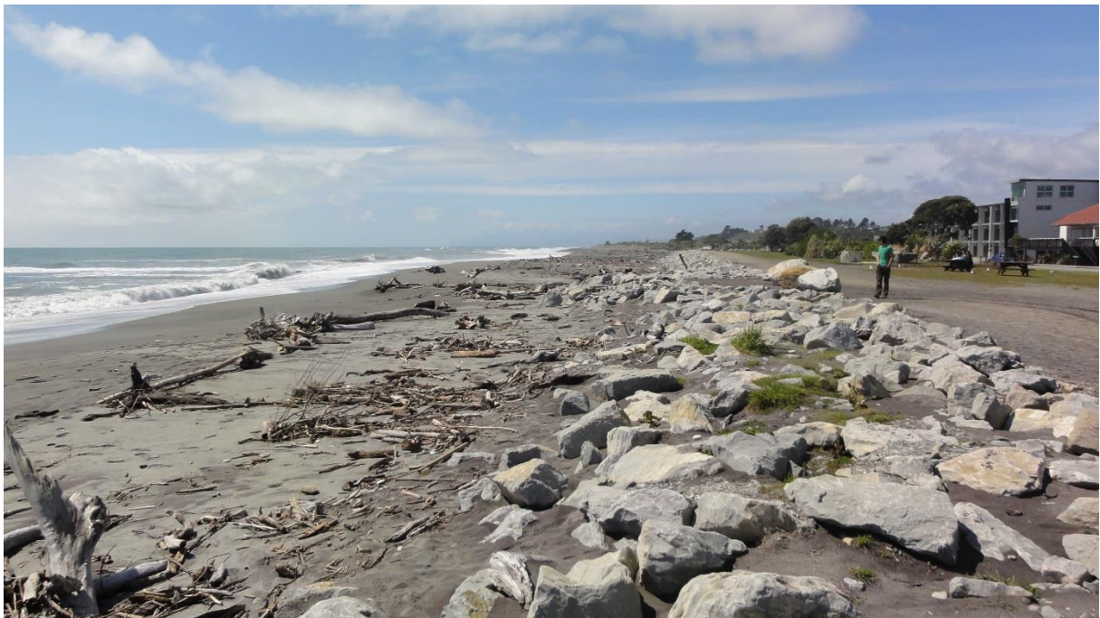
Figure 2-7: View north along Hokitika town foreshore on 28 October 2015. Note reasonably well-stocked sandy beach lapping rip-rap seawall.
